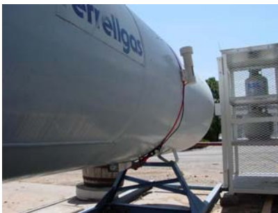
Picture 1: Installed Beta 1.0 Prototype with Telemetry Device
